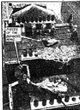
Viewing of a section taken in garden area shows the damage done to the roof of a building. (Photo after a raid.)
